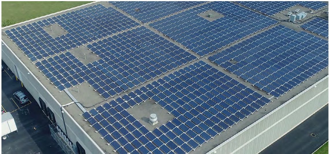
The 450kW DC Van Kirk Project.
