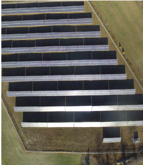
Project MC-ML81, a 600kW DC ground mount solar project.
