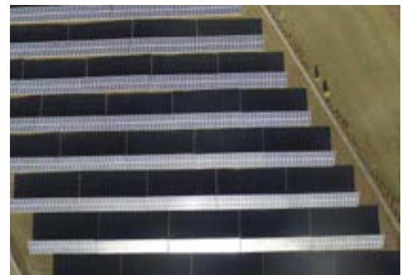
Project MC-ML81, a 600kW DC ground mount solar project.
